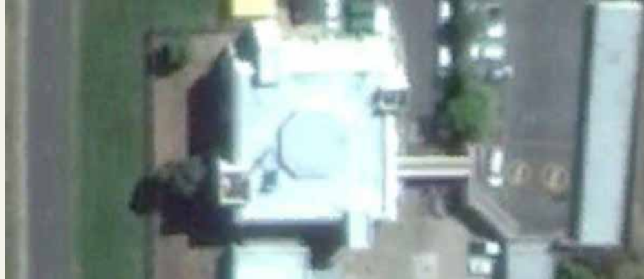
Figure 44: Roof concerns of the Electricity building
