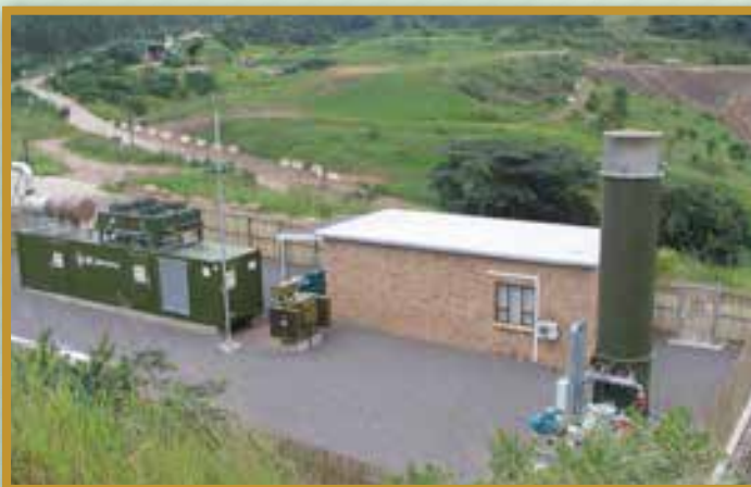
Generation unit at Mariannhill landfill site Source: eThekweni municipality
