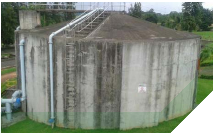
The larger 3000m 3 digester at Tzaneen WWTW
