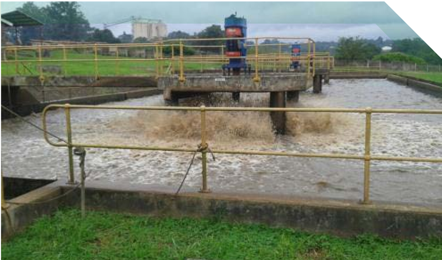
Main reactor at Tzaneen WWTW
