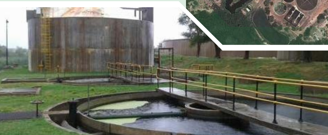
Bio-filters and Primary Settling Tanks at Kameelmond
