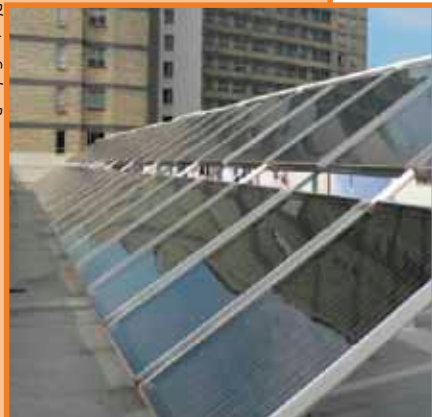
Large scale solar water heating on mid-high income Durban apartment block
