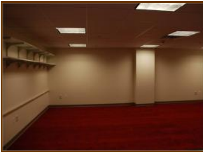
Before: A Pentagon room before Cree's LED lights were installed. (Credit: Cree)
