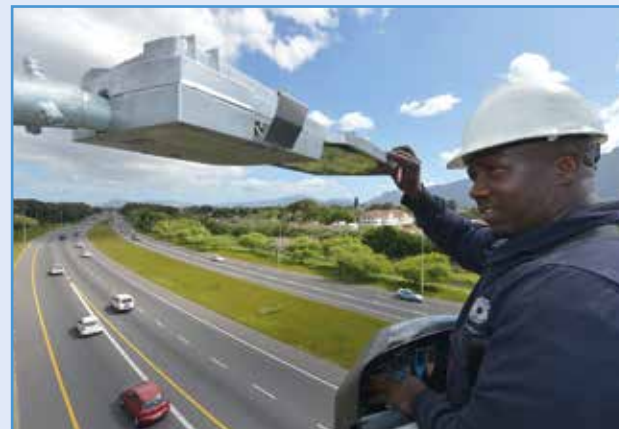
LED streetlights retrofit
