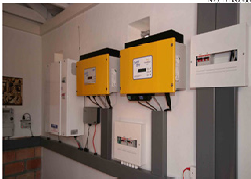
Inverters and generation control from a small-scale project installed in NMBM (2008)
