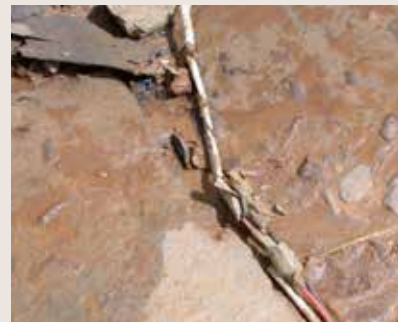
Illegal live electricity connection running across main access road and surrounded by water
