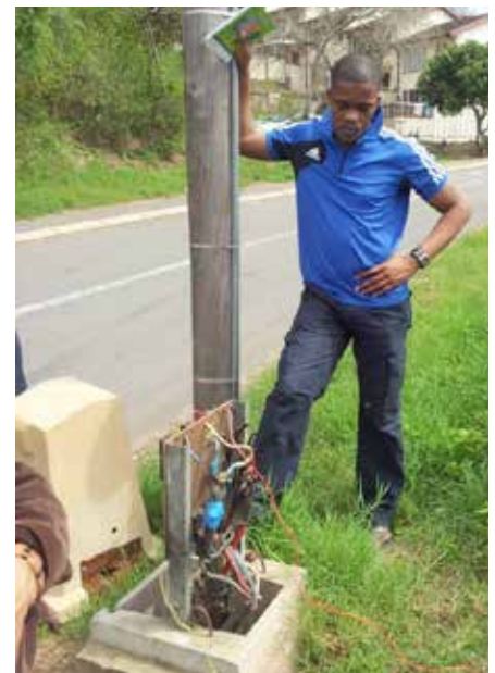
Example of an illegal electricity connection
