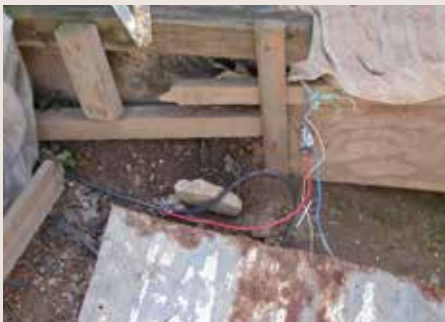
Flimsy wires and metal sheets
