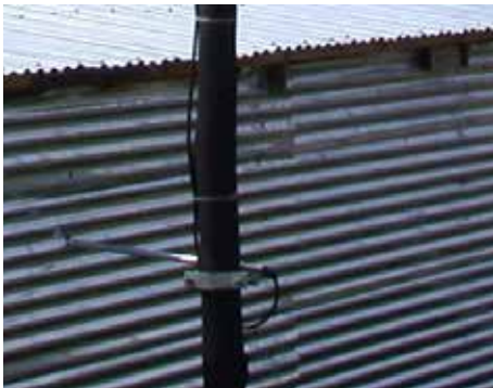
Municipal electricity connection for informal households showing service pole and prop from the pole to support the readyboard in the house
