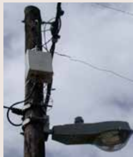
Taking illegal connection straight off the ABC
