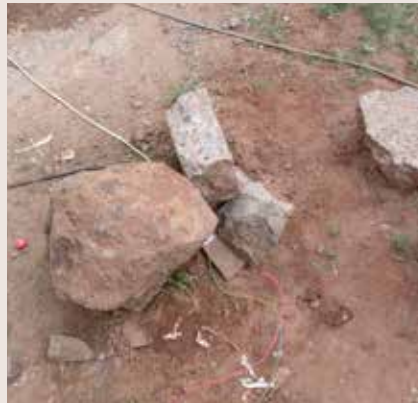
Unusual junction box (illegal wiring)
