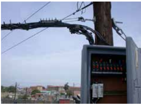
Maypole showing open 9-way box
