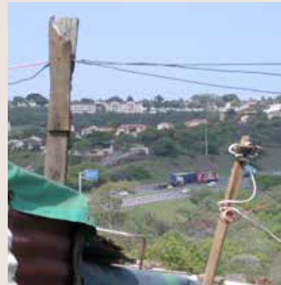
Settlements are often comprehensively reticulated, albeit illegally and unsafely
