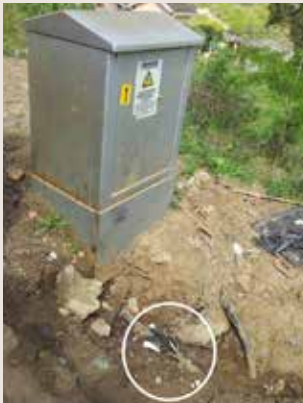
Illegal connections in a trench
