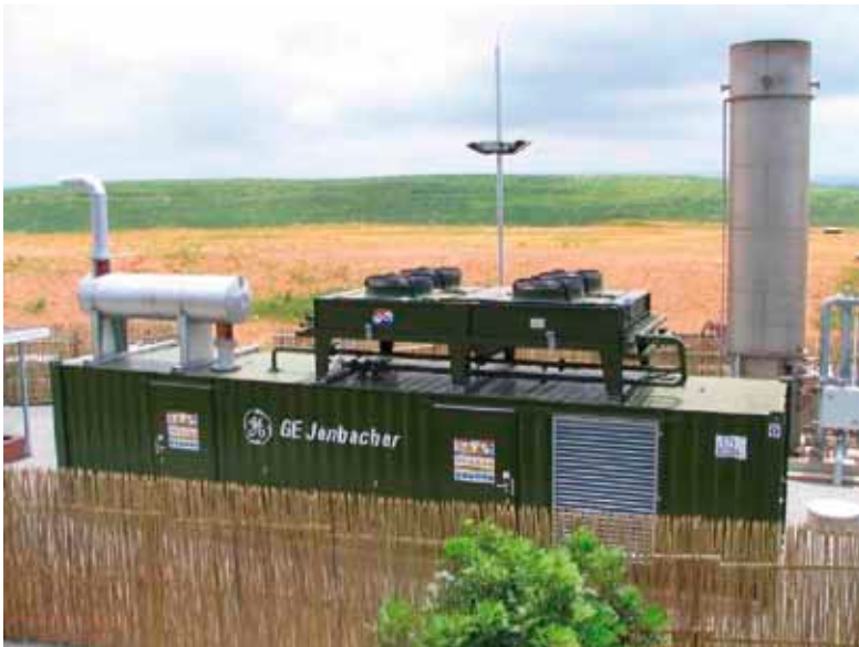
A landfill gas electricity generator at La Mercy landfill site, eThekweni
